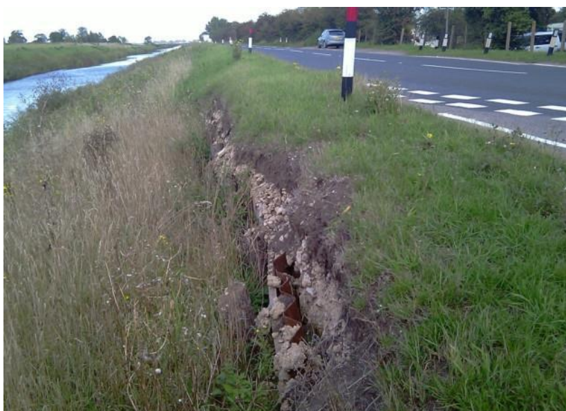
Embankment slipping at Sixteen Foot Bank near Stonea in Fenland
